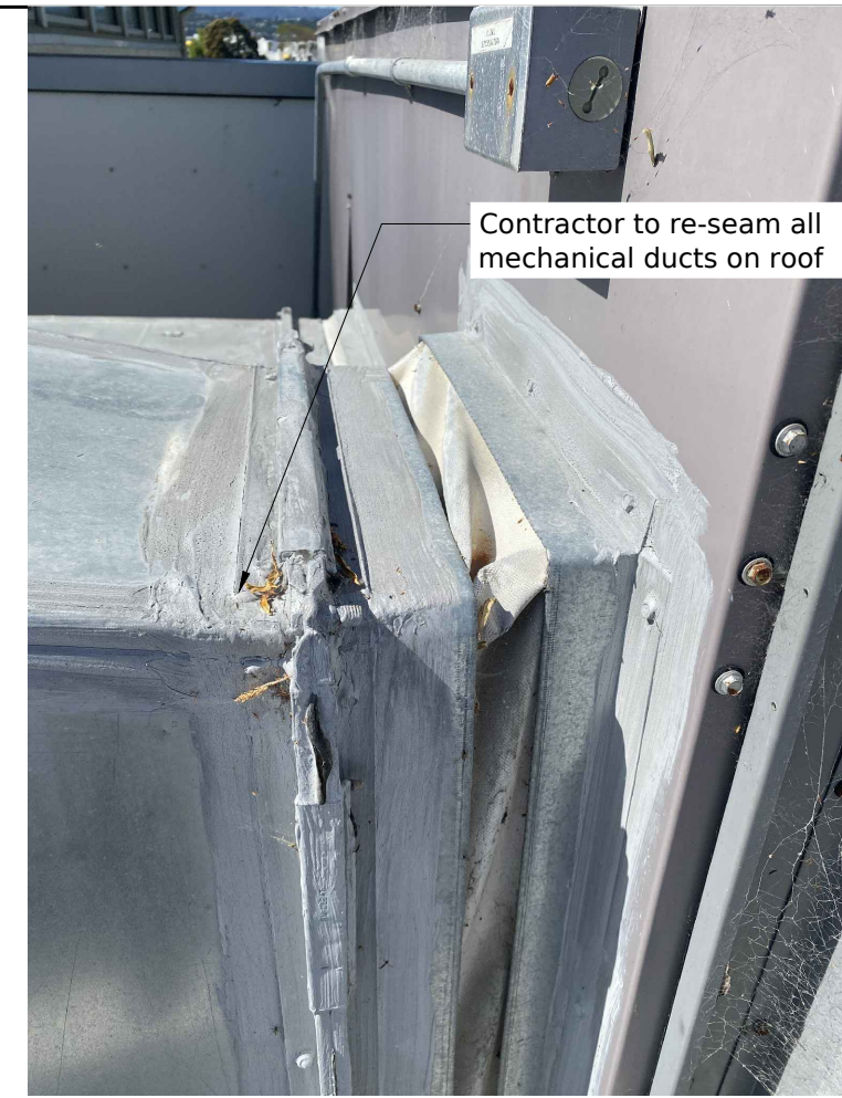
8 Mechanical Ducts Near GL 3 between GL C & D
