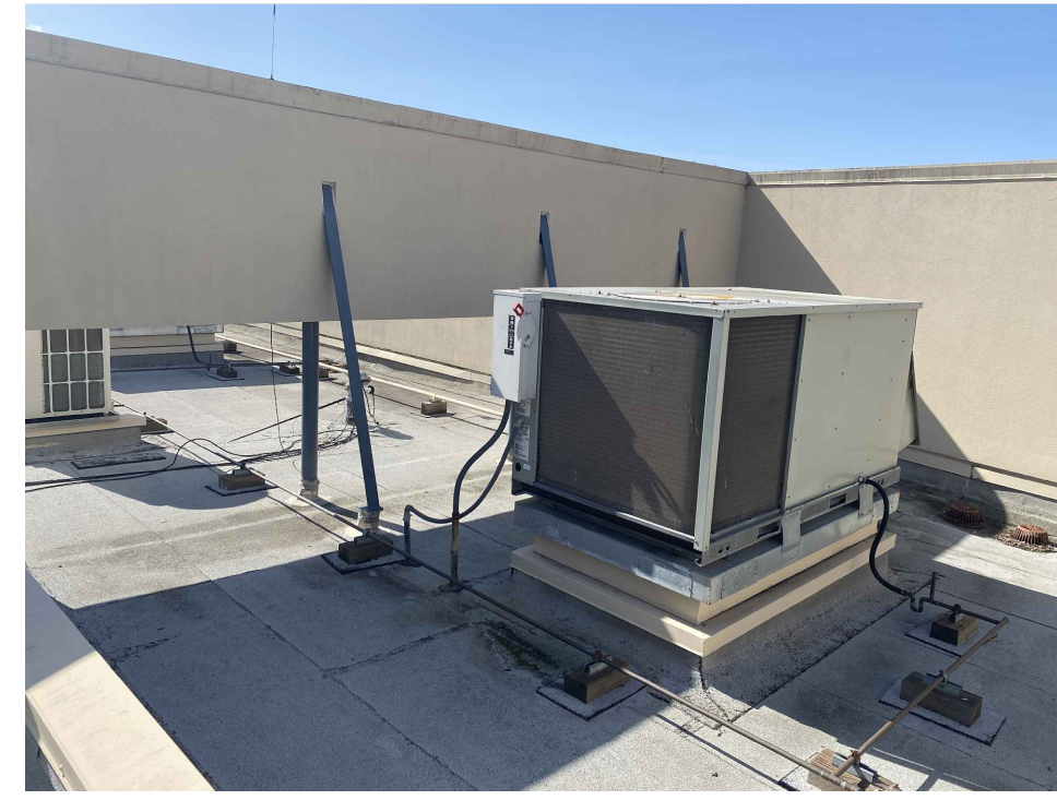
12 Mechanical equipment inside screen Northwest corner
