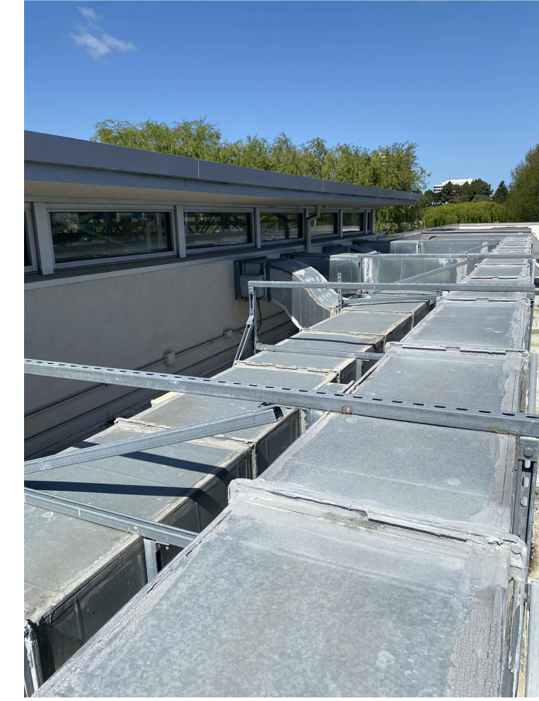
6 Mechanical Ducts Near GL D
