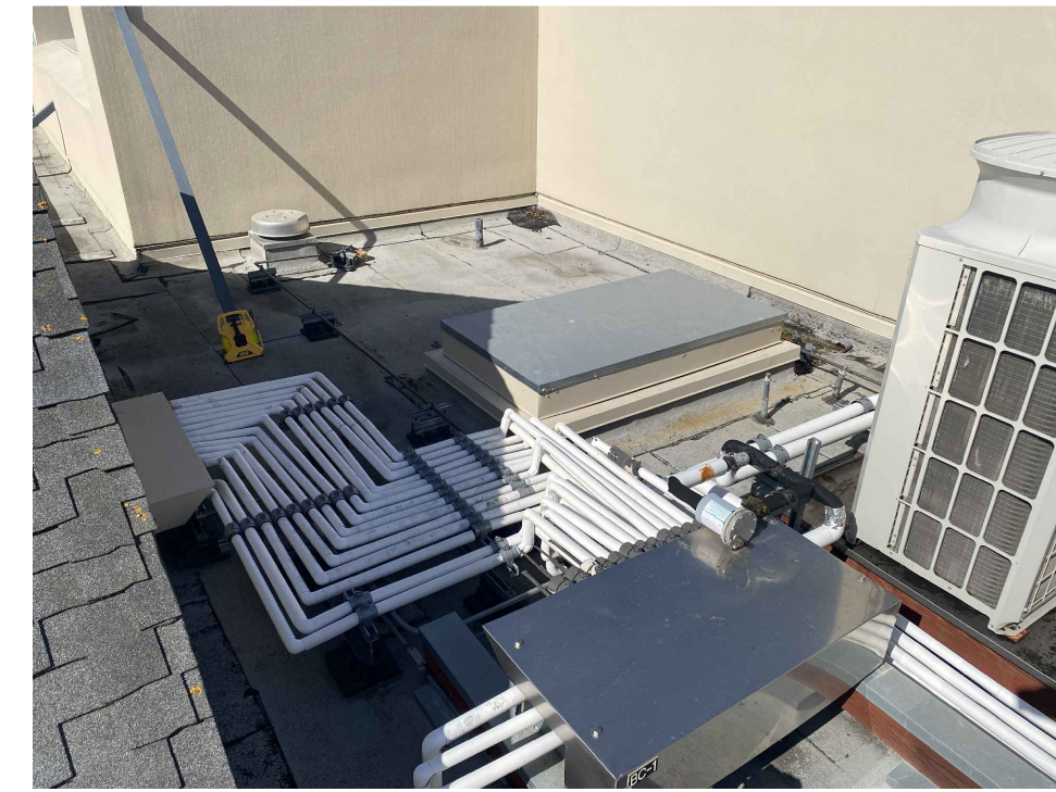
7 Pipe supports North area between GL B' and C'
