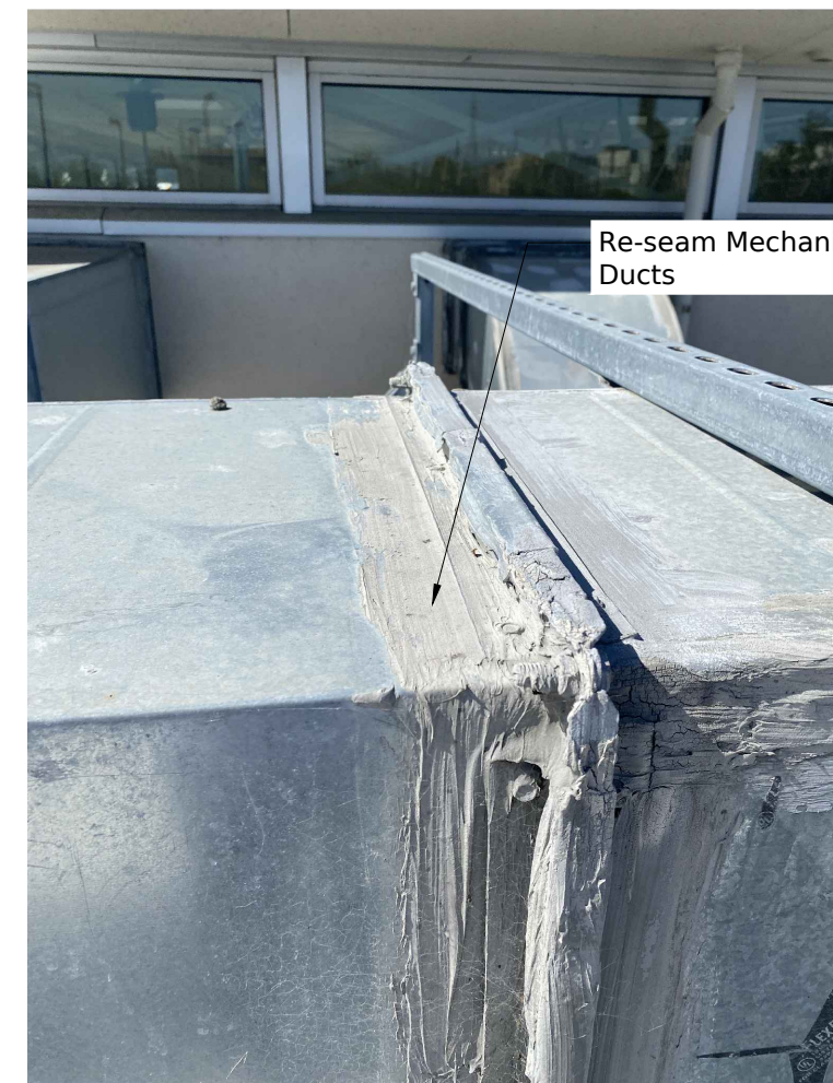
1 Mechanical Ducts Near GL D
