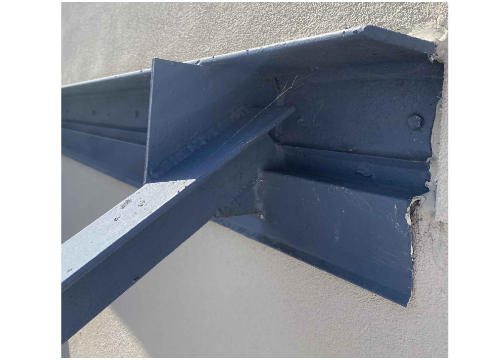
3 Angle Brace at parapet support See detail 1 for extent on East wing of roof
