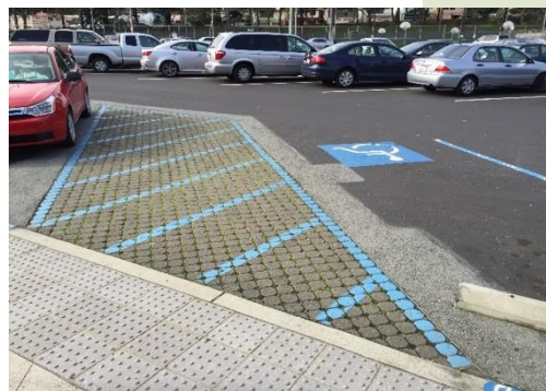
Pervious Pavement in the City of Daly City
