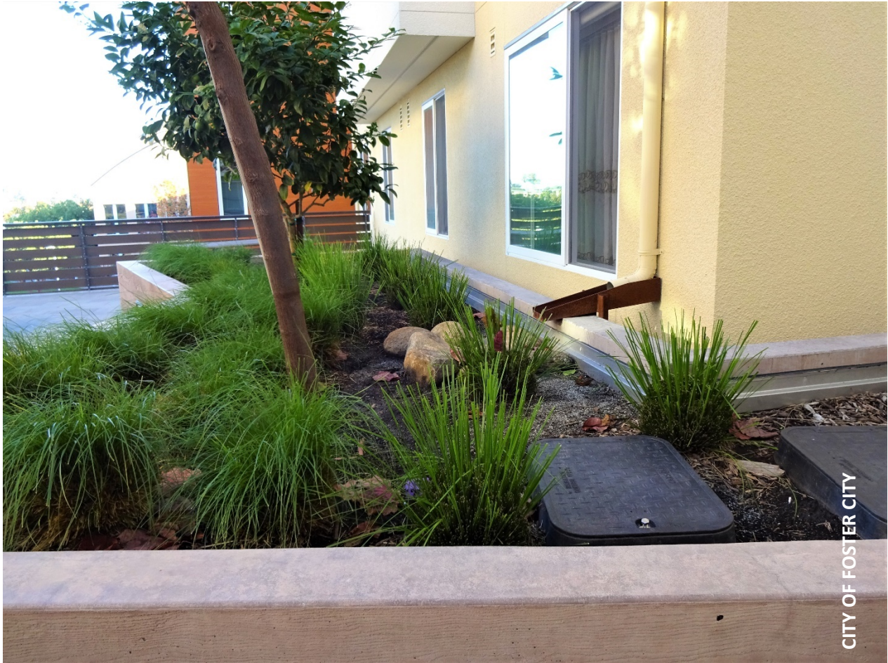
Flow-through planter located at Midpen Affordable Housing.
