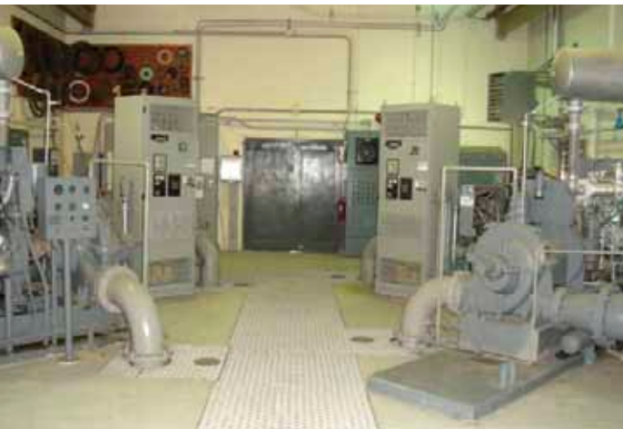
Water Booster Pump Station
